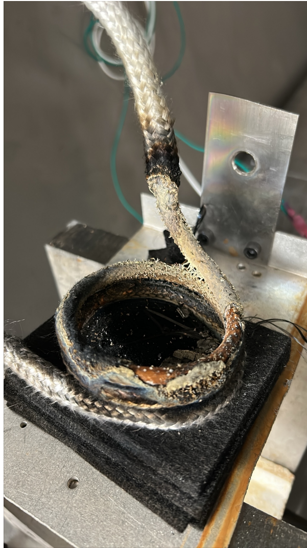
Figure 6: Melted Fiberglass insulation around the coil
